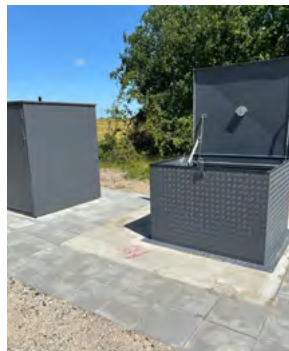
Den nye pumpestation
